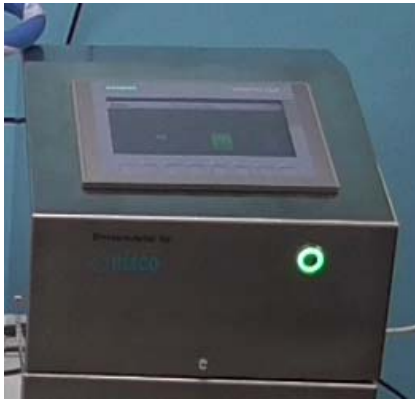
HMI control console
